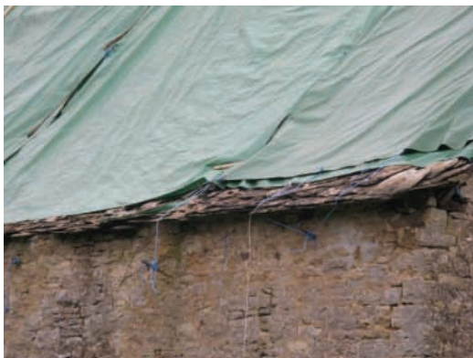
Roof tiles failing at Grade II Listed Mill House Barn: December 2008 (above and below)
