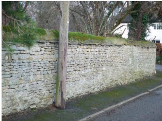
The boundary wall at Gowan Lea is a striking landmark at both Mill End and on Mill Street
